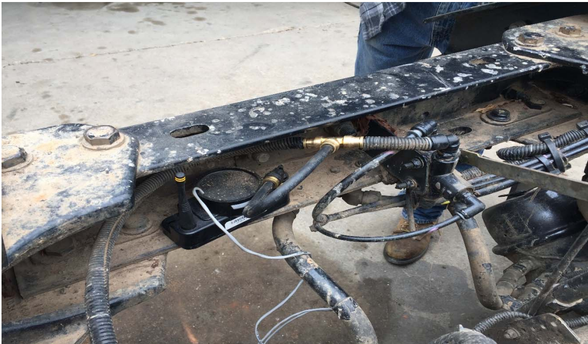
Figure 1: Air sensor installed in truck air bag suspension.
